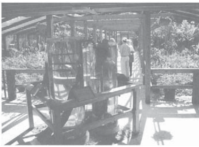
Fig. 12. Gray water for plant watering utilizing wastewater from public toilets. National Audubon Sanctuary, Cork Screw Swamp, Florida. Designer: John Todd, Living Systems Technology, Inc.
